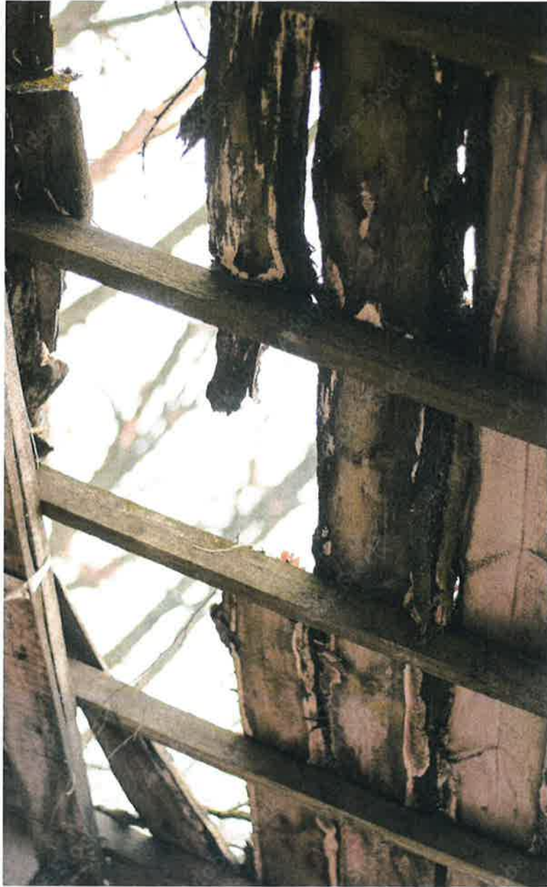
'rotten roof beams on the main house roof'
